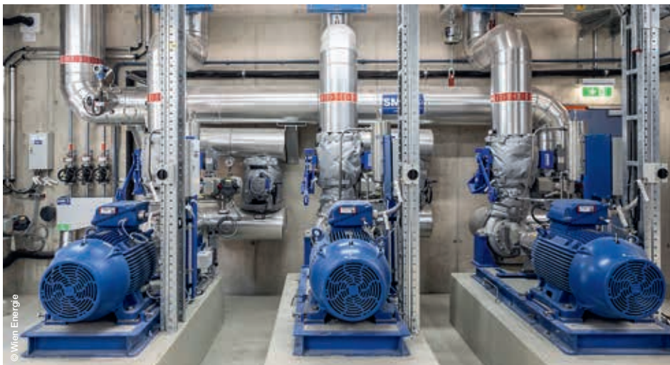
Pumps for the electric heating system including KLINGER butterfly valves
