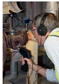
Ivan checks different points from the outside of the steam trap looking for steam leaks.
