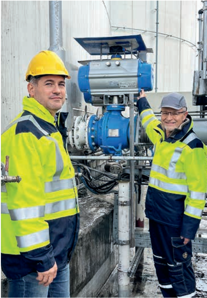
Markus Fröller and Otmar Hochreiter inspect a valve at the ELG tank farm in Linz.
